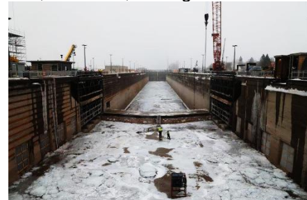
The Poe Lock dewatered to undergo critical maintenance over the winter month. Credit: U.S. Army Corps of Engineers.
